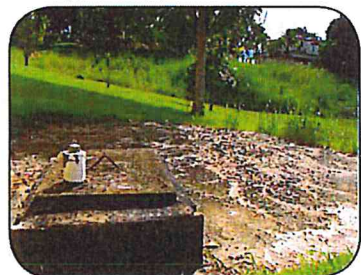
Keep septic tanks sealed.
