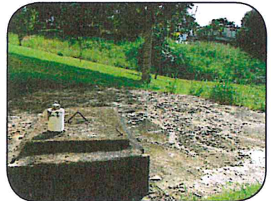
Keep septic tanks sealed.
